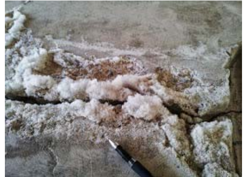
Efflorescence, salts being “purged” out of the slab by the action of the CMW
